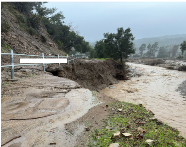
Ventura River bank eroded and broke one of two sewage lines the first week of January 2023 at San Antonio Creek. Photo credit: Rick Reid
