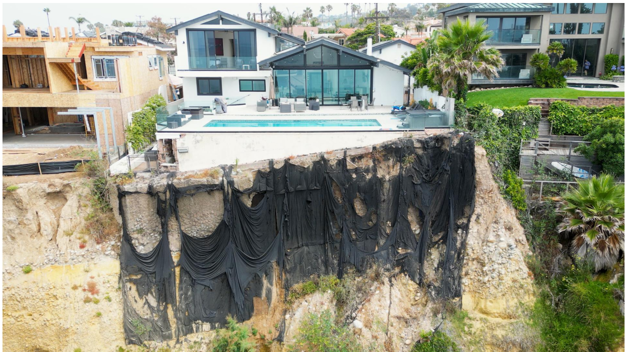
This July 15, 2023 photograph shows the current, dilapidated state of the tarp
