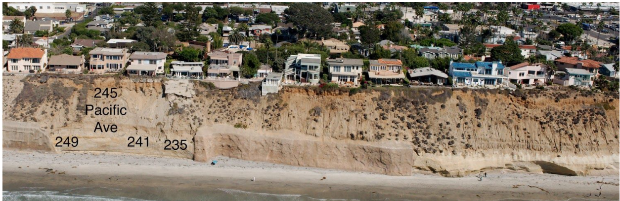
Going south from Tide Park (475 Pacific Ave) to 235 Pacific Ave and beyond
