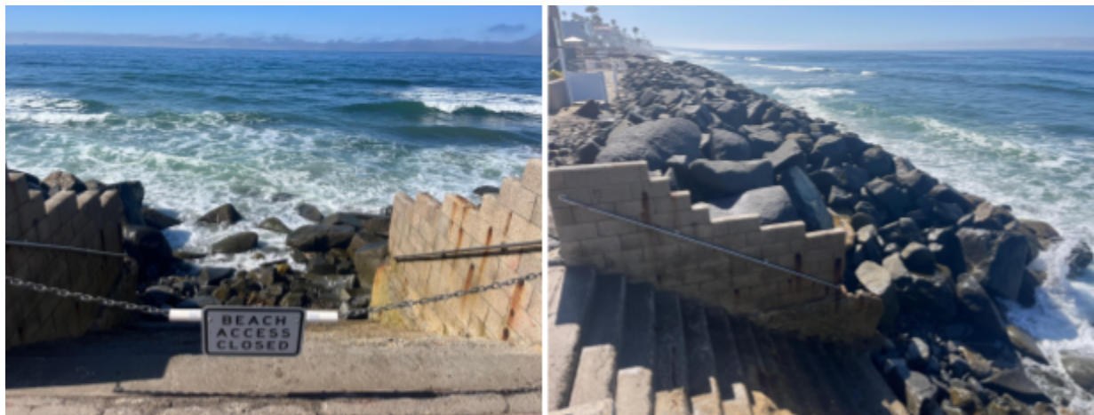
Left: Hayes Street vertical access is currently closed and unsafe. Right: lack of lateral access into project area (3.5 ft tide).
