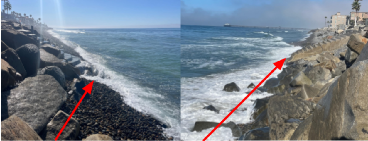
The private staircase at 917 S Pacific, partially submerged at a 3.5 foot tide. The private staircase at 1023 South Pacific, partially seaward of a 3.5 foot tide.
