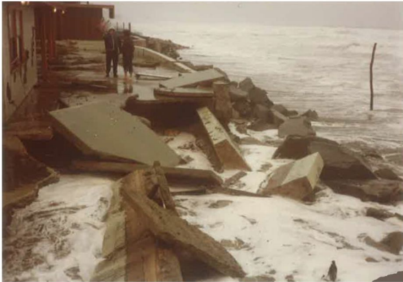
Coastal Damage following 1983 Storm
