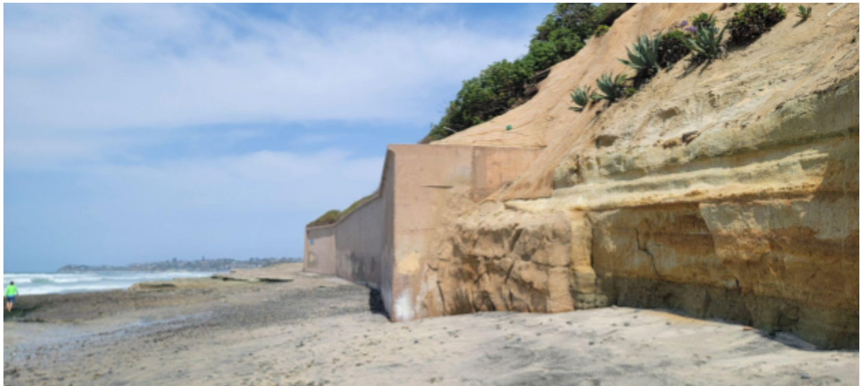
Passive Erosion at Steinberg Seawall as observed in March 2025. Note the continued erosion of the adjacent area to the south of the seawall. Also note the presence of wave driven cobble immediately shoreward of the seawall.
