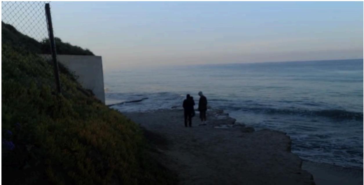
Beach access along bedrock platform at Steinberg Seawall as observed in January 2022. This access connects the southern portion of the State Beach to its parking lot and pedestrian access from South Coast Highway 101.
