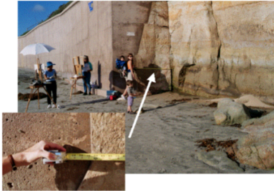
Passive Erosion at Steinberg Seawall as observed in approximately 2001
