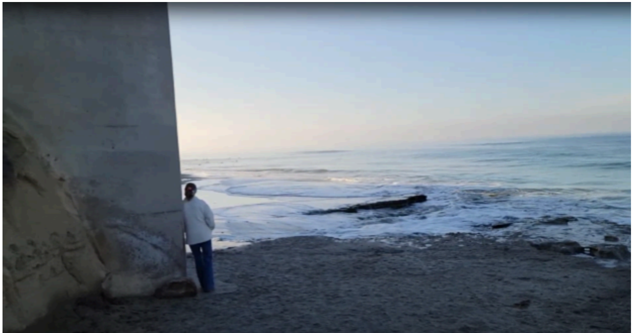
Flooding of beach access to South Cardiff State Beach and front of Steinberg Seawall as observed on December 23, 2022.
