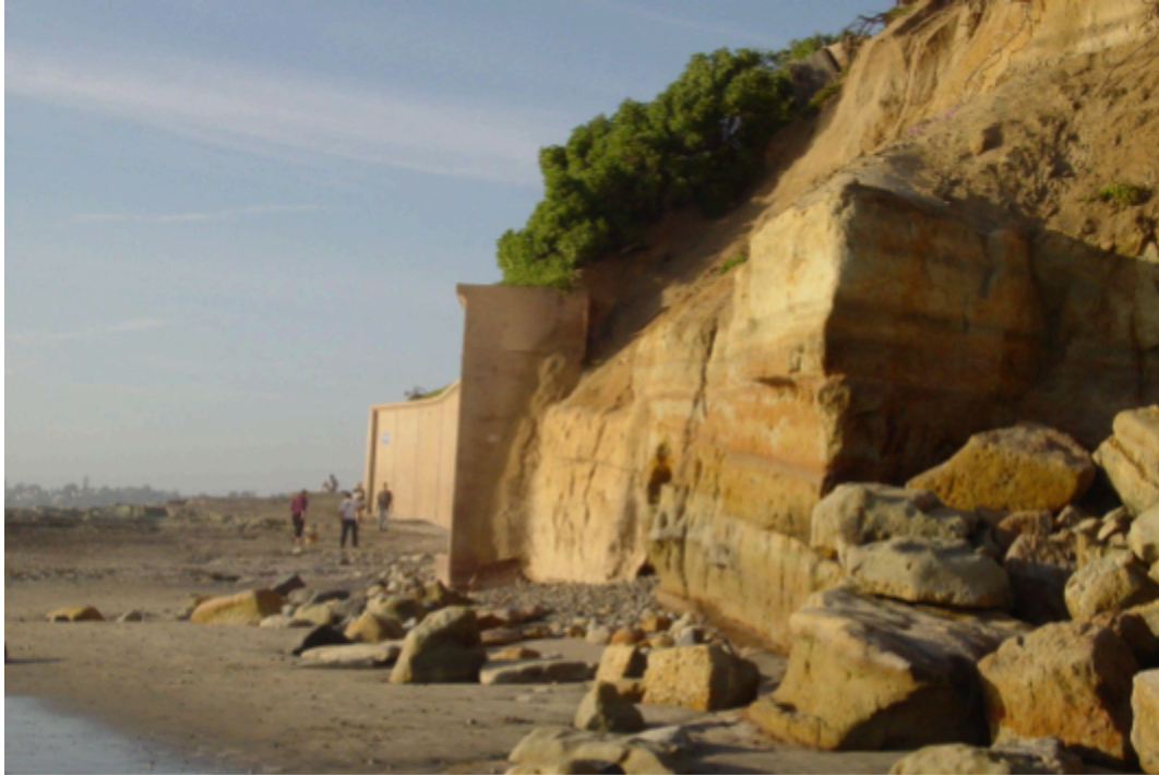
Passive Erosion at Steinberg Seawall as observed in 2005. Note the presence of eroded blocks and an already constructed fill and return wall.
