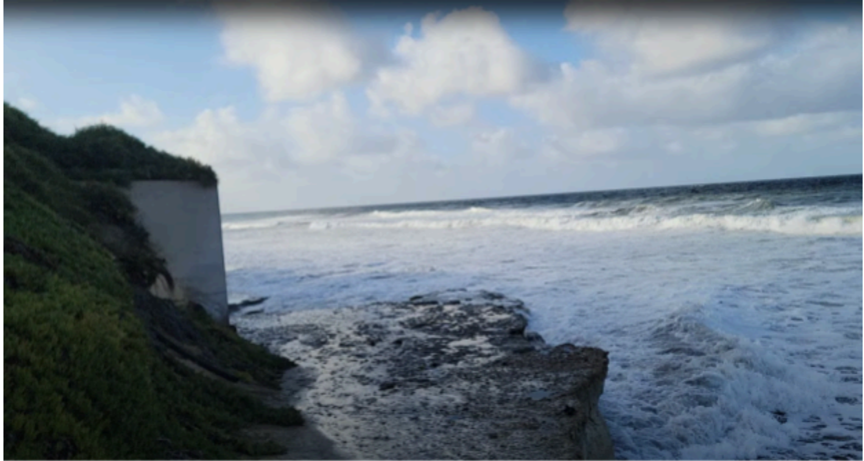
Flooding of beach access to South Cardiff State Beach and front of Steinberg Seawall as observed on November 15, 2024.
