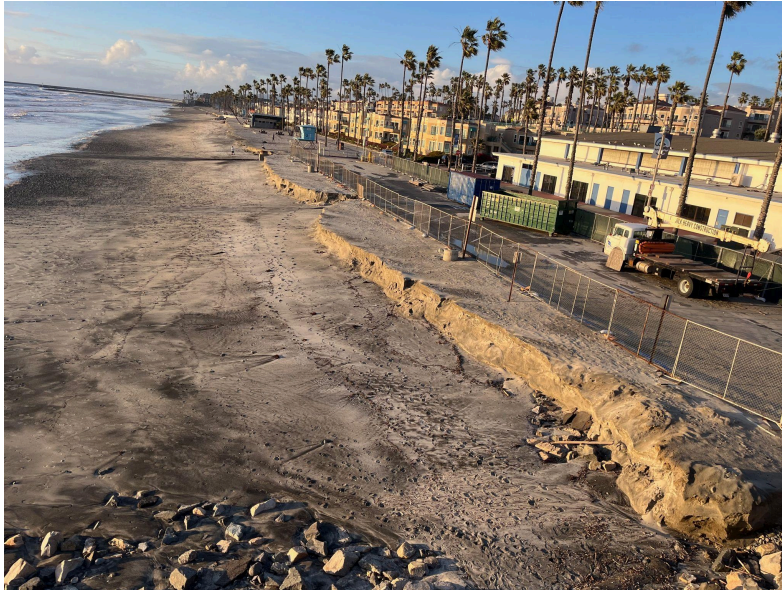
February 2024 - Beach scarping comes perilously close to a parking lot, The Strand, and the Junior Seau Community Center (part of the Beachfront Improvements Project). This beach relies on annual Harbor dredging to remain viable in the near-term. Photo taken at deep low tide, facing North from the Pier.
