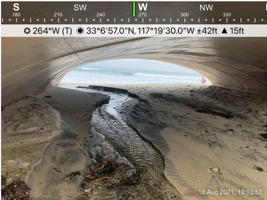
Photo 29. The culvert at southbound Carlsbad Boulevard has accreted beach sand and a low flow trickle drained Encinas Creek to the ocean outlet at the time of the August surveys.
