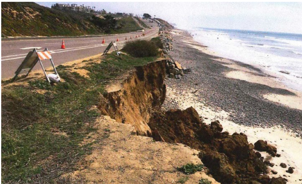
Figure 3-4. Erosion along Southbound Carlsbad Boulevard near Encinas Creek (Photo taken 3/17/2016 by City of Carlsbad)
