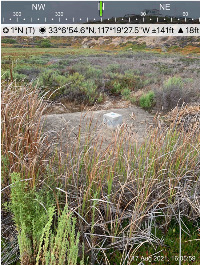
Photo 6. Pickleweed marsh south of Encinas Creek extended up to a concrete pad with a marker indicating the placement of the outfall pipe. Unusual patterns of dead vegetation and wetland plants such as cattails around the pad may indicate that the outfall pipe is another source of hydrology in the Study Area.
