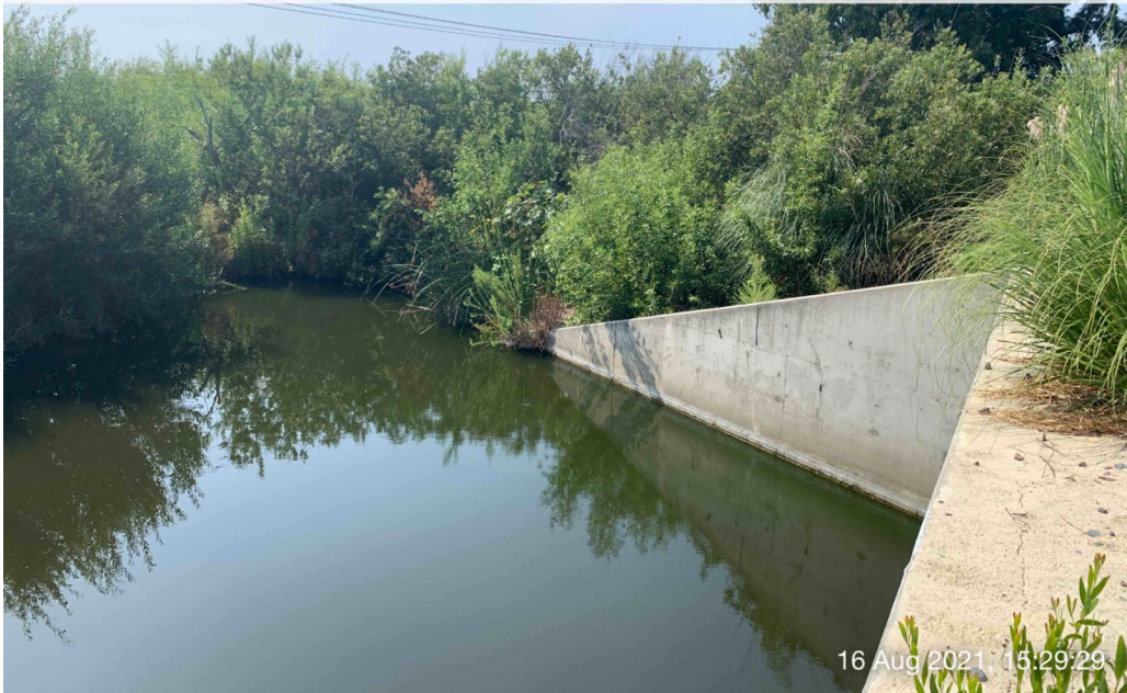
Photo 24. A large scour pool occurs at the outlet of the large culvert under Avenidas Encinas.
