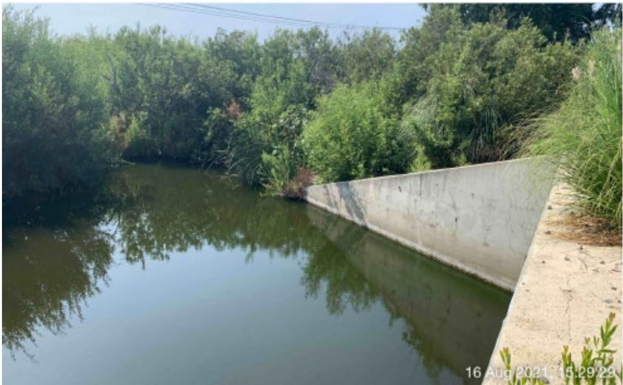
Figure 3-6. Large scour pool at the outlet of the large culvert under Avenidas Encinas
