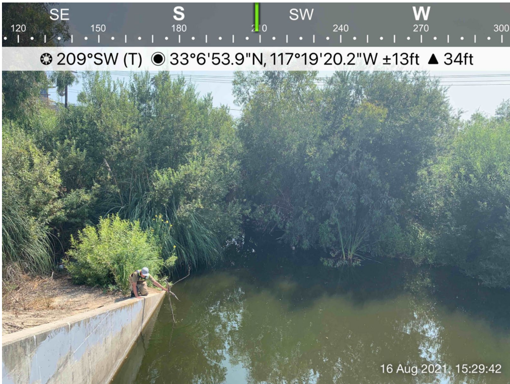
Photo 25. The large scour pool appeared to be deep at the center, and depth at the thalweg is unknown.
