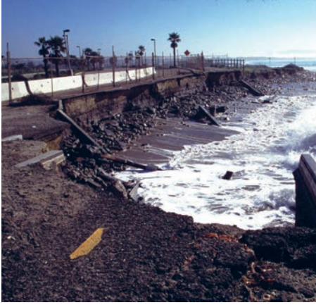
Damaged bike path at Surfers' Point prior to the Surfers' Point Managed Shoreline Retreat project.
