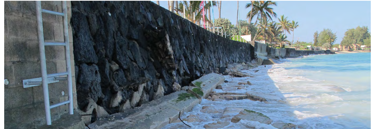
Beach loss due to shoreline hardening and seawalls in Mokulē’ia. Photo: Hawai’i Department of Land and Natural Resources, Office of Conservation and Coastal Lands
