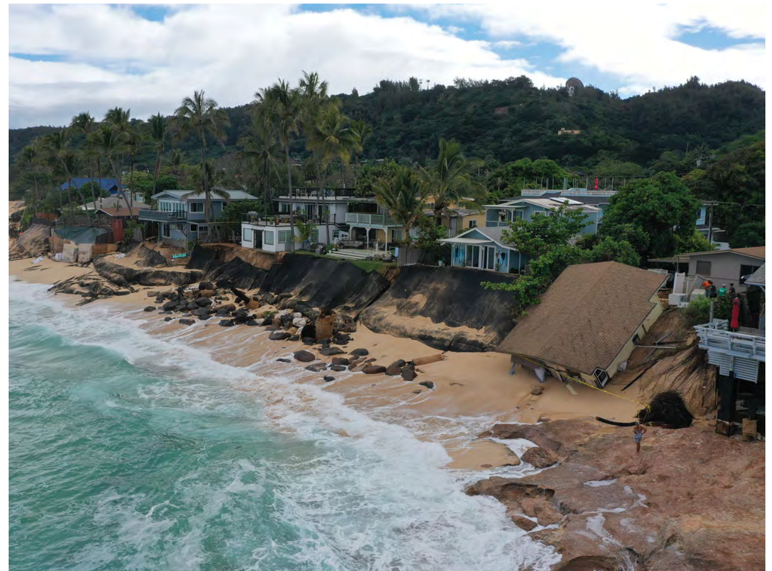
Collapsed home, tarps and other temporary erosion control measures, and impaired beach access between Rocky Point and Sunset Beach Park, North Shore, 2022. Photo: Shellie Habel, Sea Grant/DLNR
